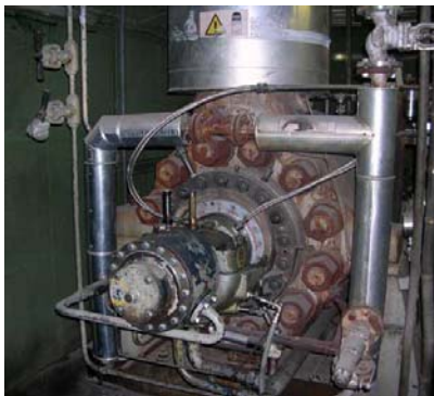
Pumps, at the “Andrea Palladium” thermal power station
